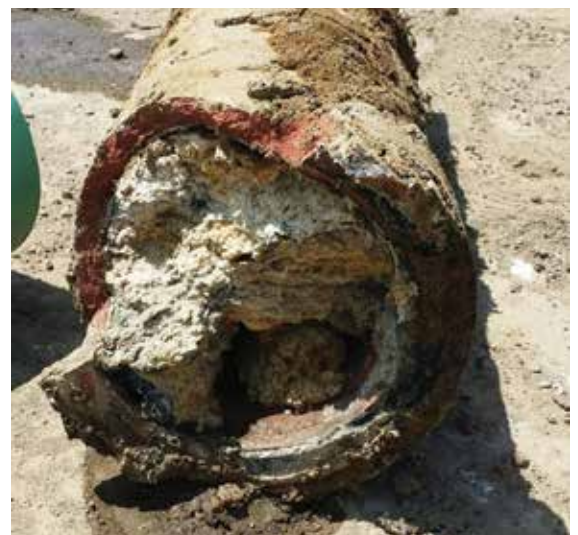
This sewer main was found to be completely clogged with grease in Madison, SD.
